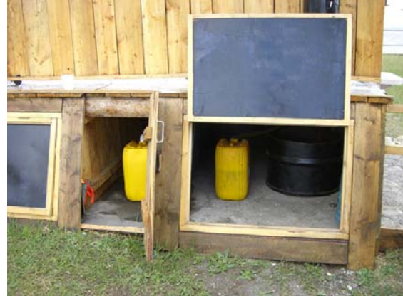
Photo 3: Back view of the ecosan toilet, close-up
